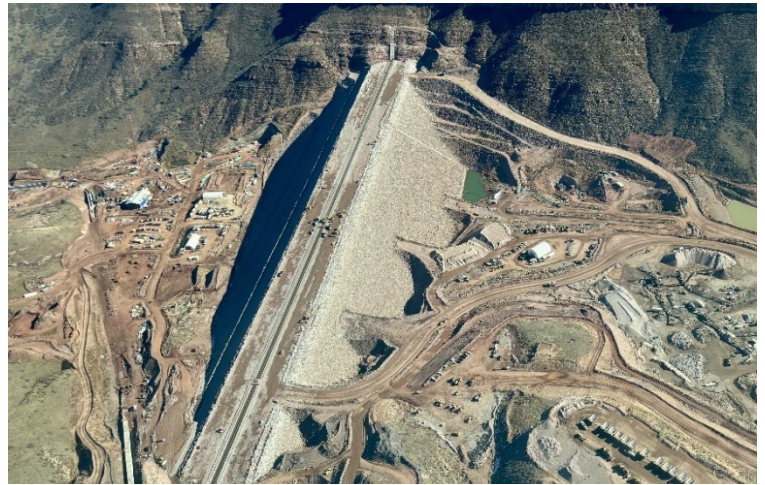
Construction of Chimney Hollow Reservoir is nearing completion and is anticipated to be complete in summer 2025. This shows the main dam.
